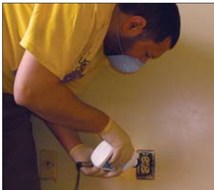
Tempo 1% dust was applied to several areas, including electric outlets.
